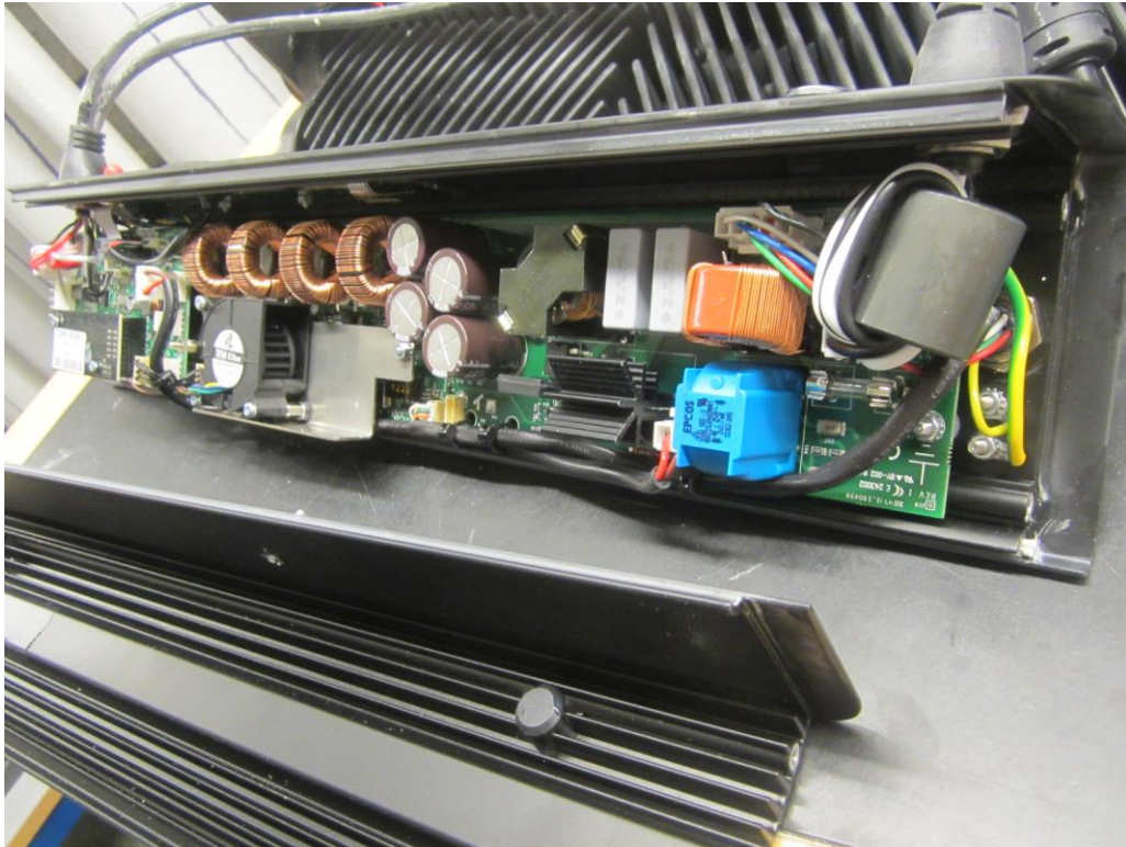
Photo 9. IP6X No dust observed inside the P-5 Wash Light.
