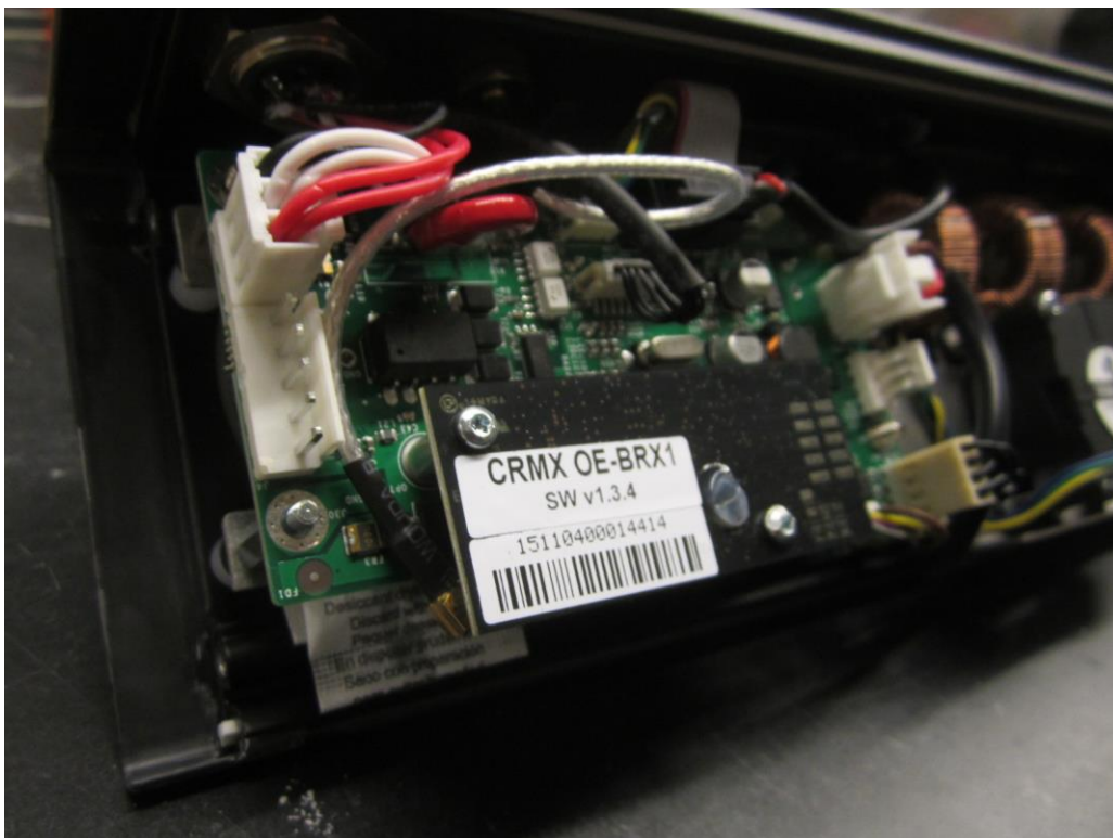
Photo 10. IP6X No dust observed inside the P-5 Wash Light.
